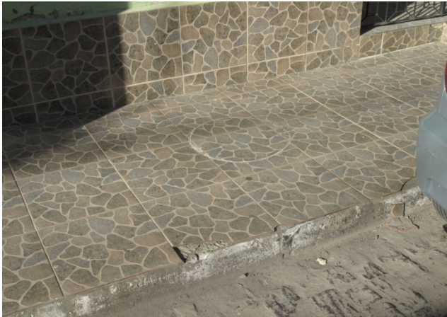
Photo 5. Manhole cover that has been incorporated into the sidewalk in Salvador
