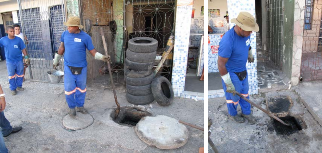
Photo 9. A condominial sewer line on public land in Salvador: a team from EMBASA carrying out maintenance using hand tools
