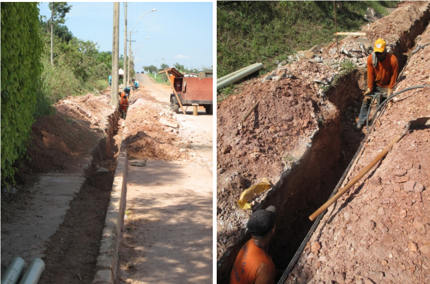
Photo 8. CAESB contractors digging trenches for sewer lines in a residential district of Brasilia
