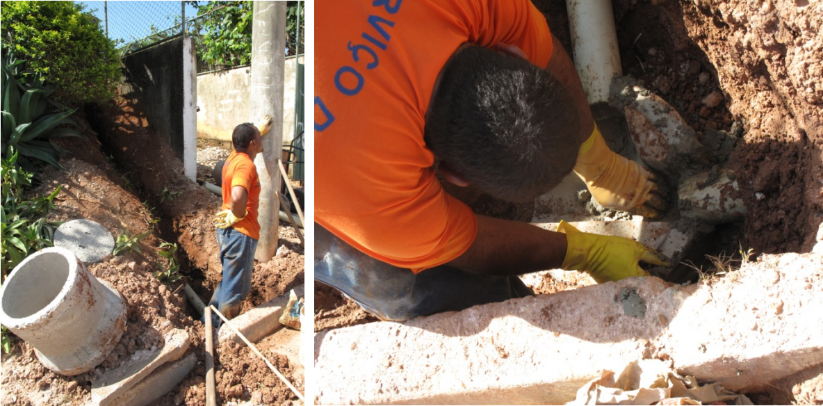
Photo 7. CAESB contractors laying a connection manhole in a residential district of Brasilia
