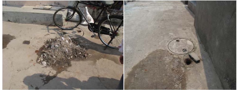
Photos 3 and 5: Sludge from the manhole emptied into the street, manhole opened to enable stormwater drainage and broken pipes in Ramagundam, India
