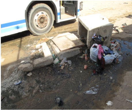
Photo 4: Broken manhole blocked by solid waste that is overflowing into the street in Rufisque (Senegal).
