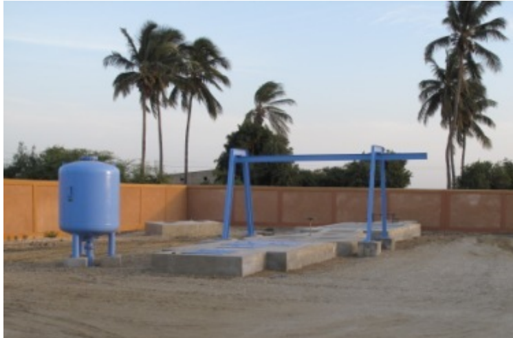
Photo 1: Lift station in Saint-Louis, Senegal (large capacity as it also receives effluent from the conventional sewer system).
